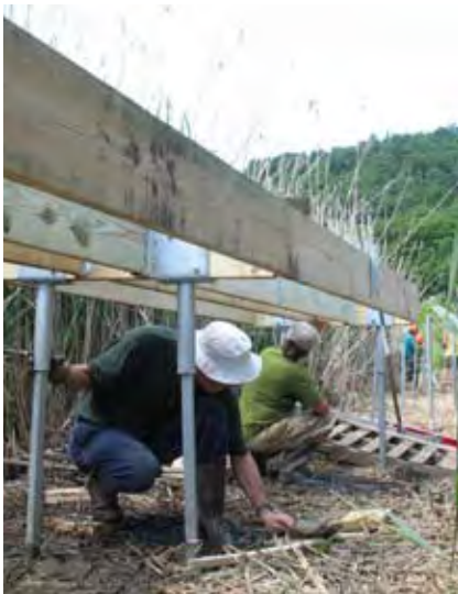
Image 50. Volunteers constructing a boardwalk with steel helical piers to minimize ground disturbance.
