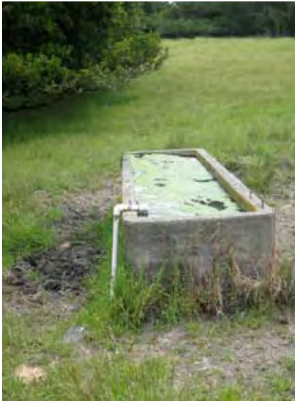
Image 20. Typical water trough in need of repair. PHOTO: LISA BUSH
