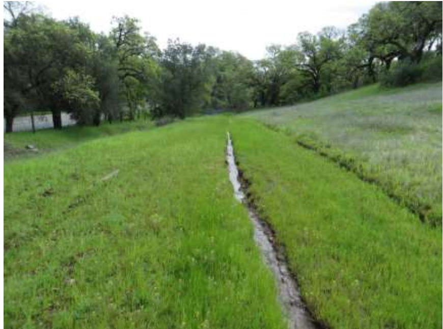
Concentrated flow/erosion along trail.
