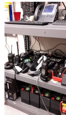
Two-way Radios – average weight 2 lbs. Staging area in workshop Smaller Batteries stored at 4-inch height
