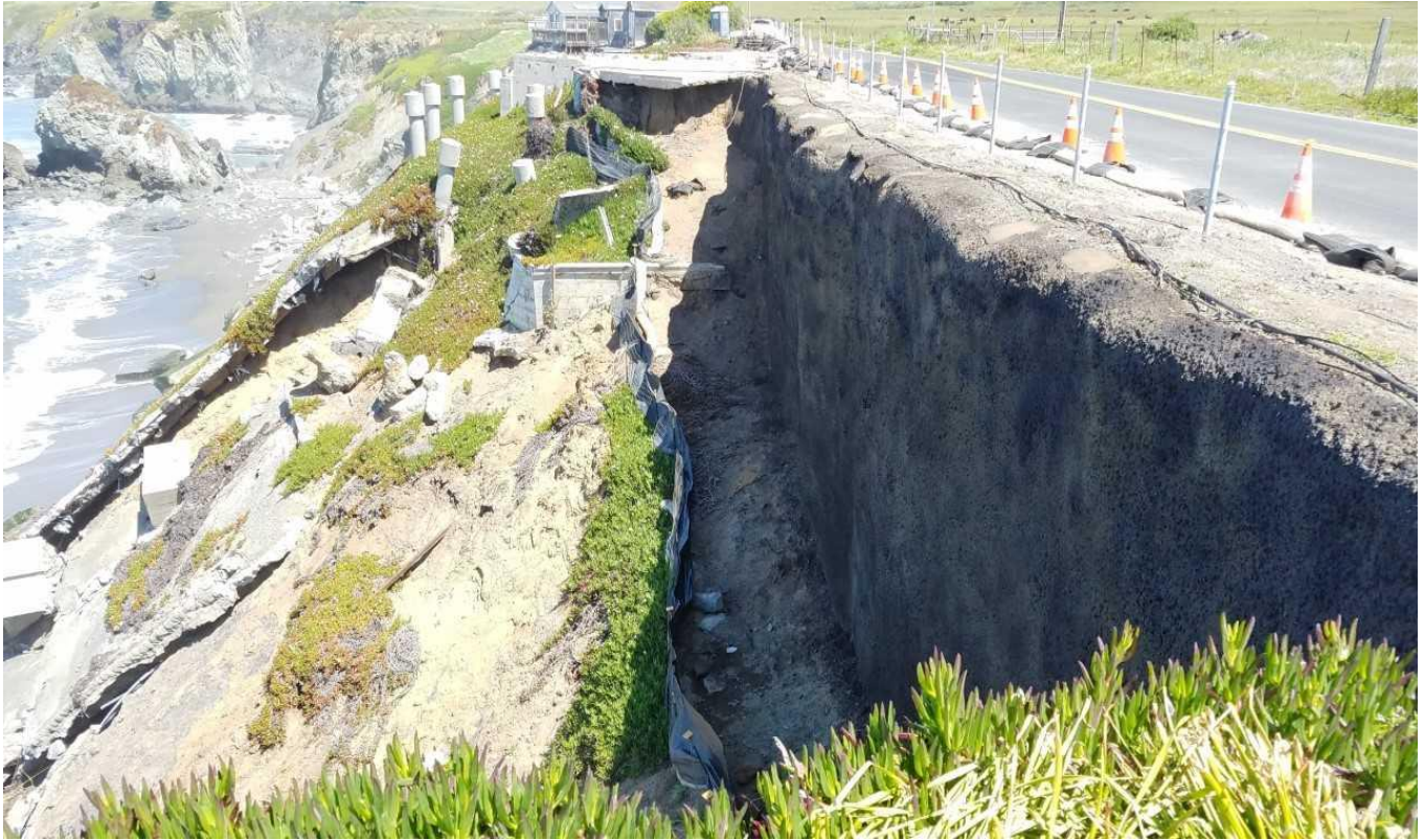
Caltrans 2017 Shotcrete Wall and Sluffing Debris along Highway 1, Bluff Face and Shoreline
