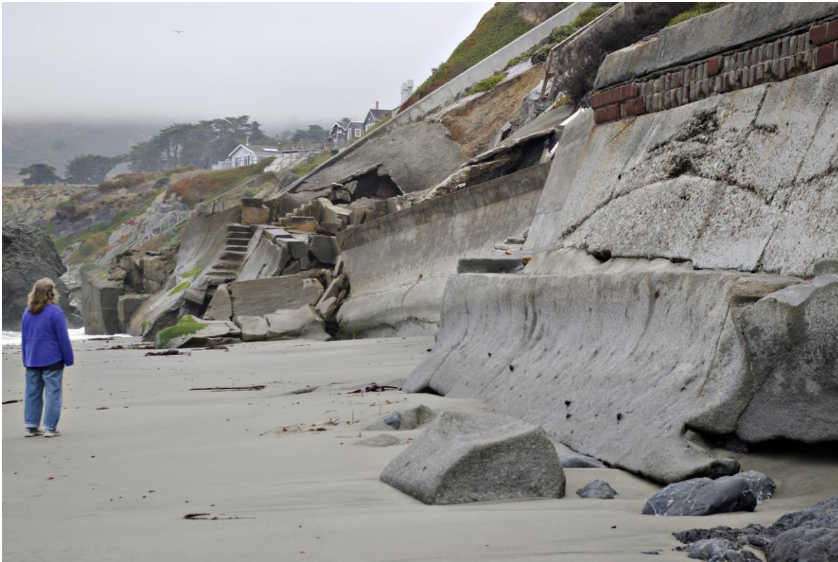
Shoreline perspective of debris along Gleason Beach bluffs Source: Sonoma County
