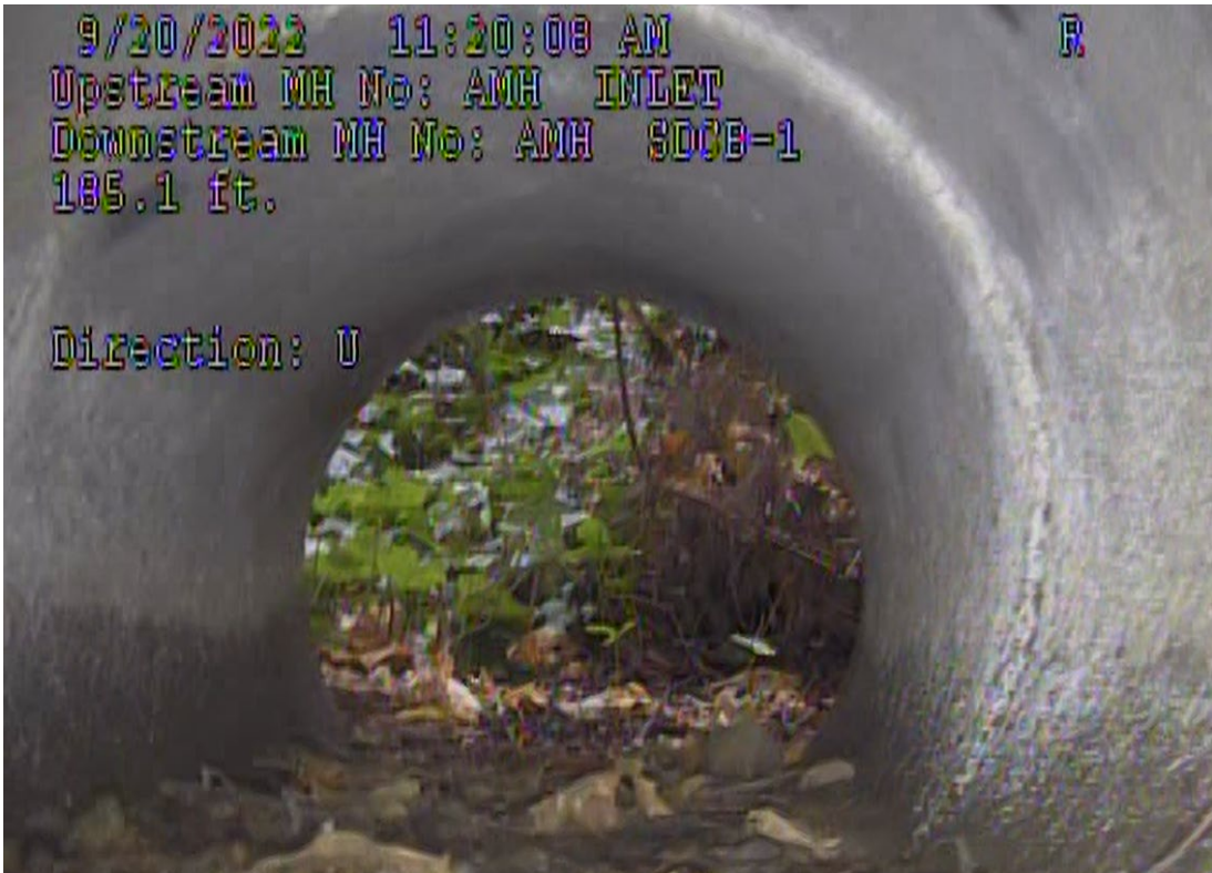
Figure 5-30: Overgrowth and Sediment Accumulation at Upstream end of 6 th Street (24-inch RCP)
