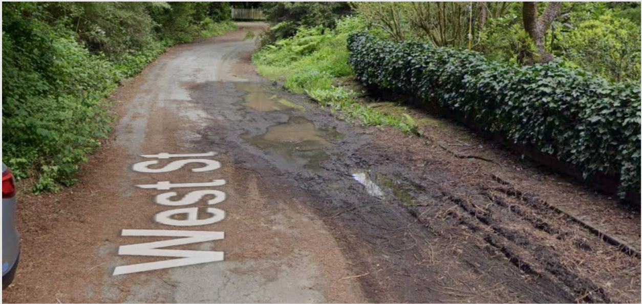
Figure 5-5: Ponded Water and Sediment Buildup on West Street (Between Post Office and East St)
