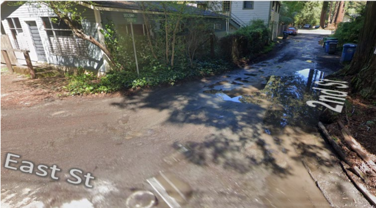
Figure 5-4: Ponded Water at East Street and 2 nd Street
