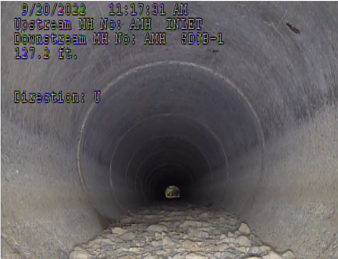
Figure 5-29: Rock and Sediment Accumulation in 6 th Street RCP
