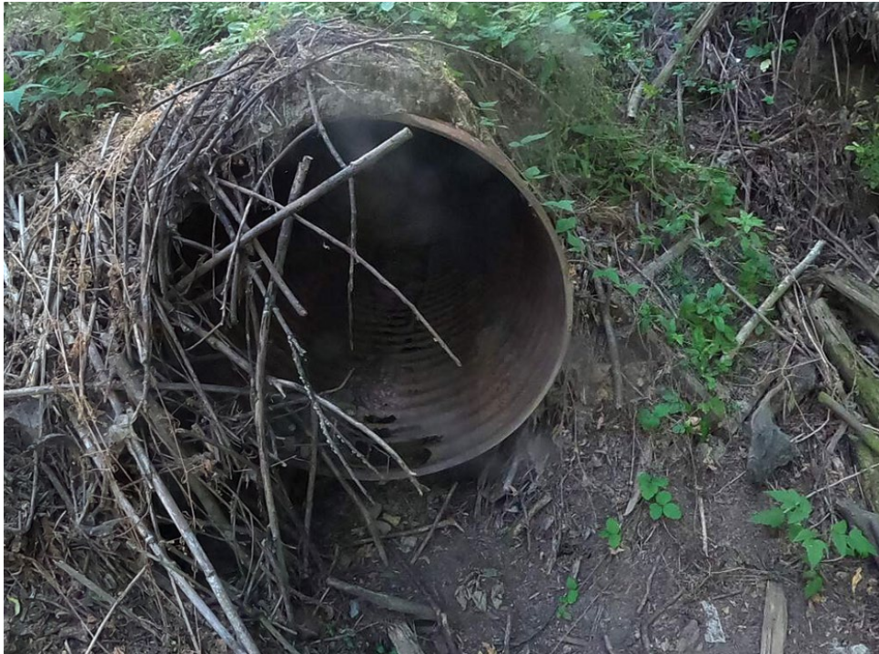
Figure 5-10: Southern Pipe System Outfall (From 6 th Street).
