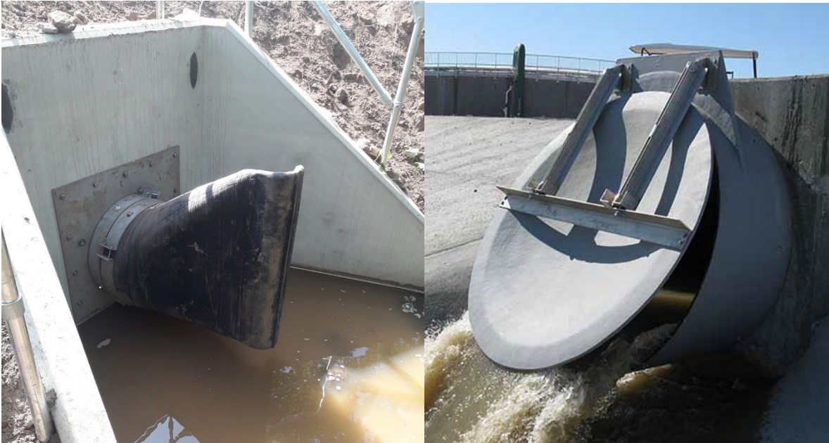
Figure 5-11: Tideflex (Left) and Flap Gate (Right) Non-Return Valves on Outfall Ends
