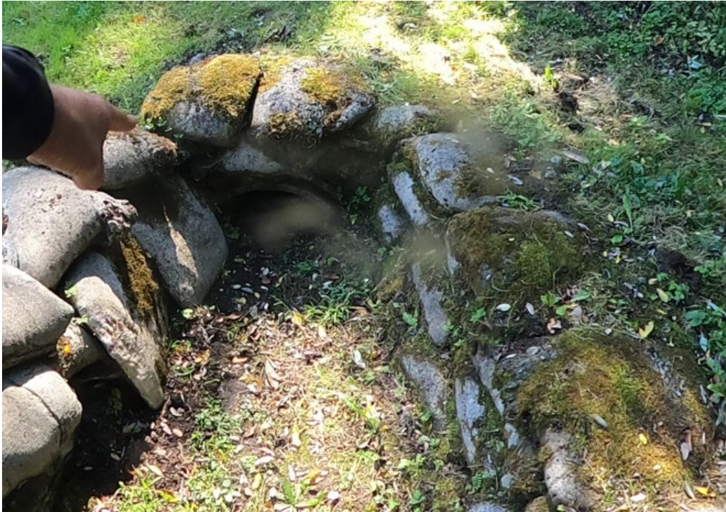
Figure 5-26: 4 th Street Outfall Daylight Section Sediment Buildup
