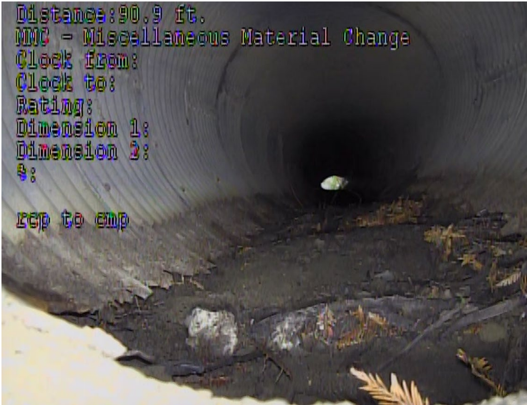
Figure 5-31: Corroded CMP Bottom at Transition from RCP to CMP (6 th Street Outfall)
