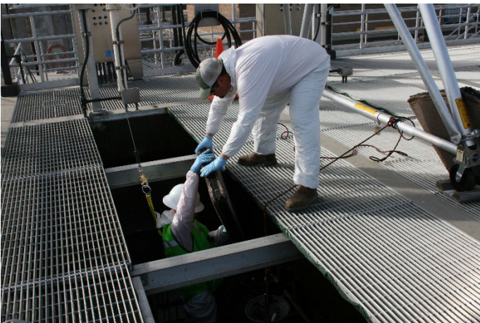
Example Photo 6: Filter Removal and Confined Space Entry Safety Analysis/SOP Development/Safety Training
