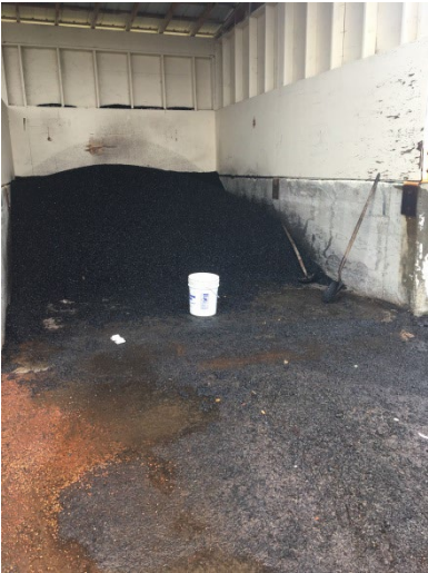
Cold Mix Asphalt Repair Material Shovel and 5 Gallon Bucket for Pot hole repair
