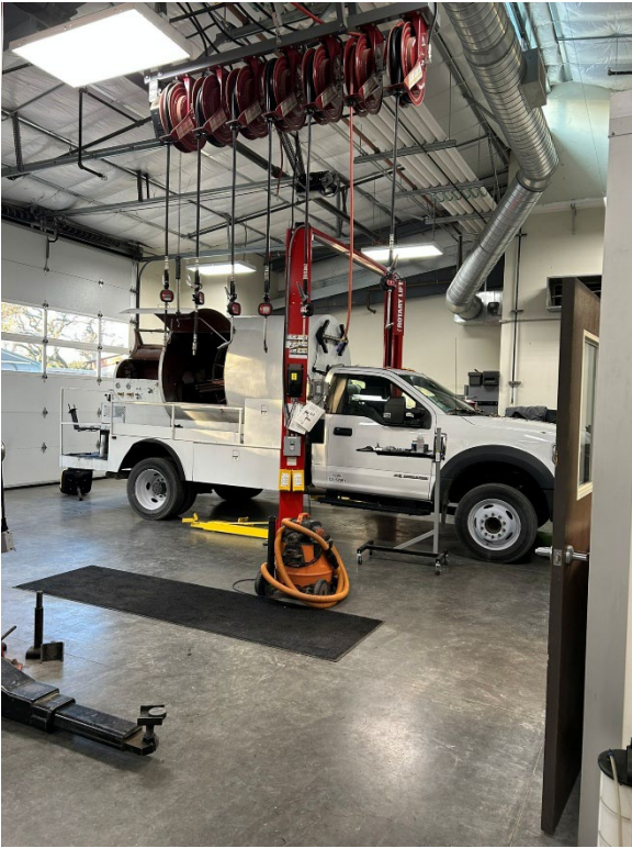
Light Equipment/Vehicle Service Bay - Easy access to hoses over-head
